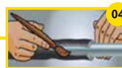
04 Applying a very thin layer of special adhesive to the edges to be joined
