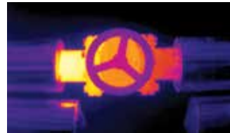
Thermal camera view of the uninsulated valve
